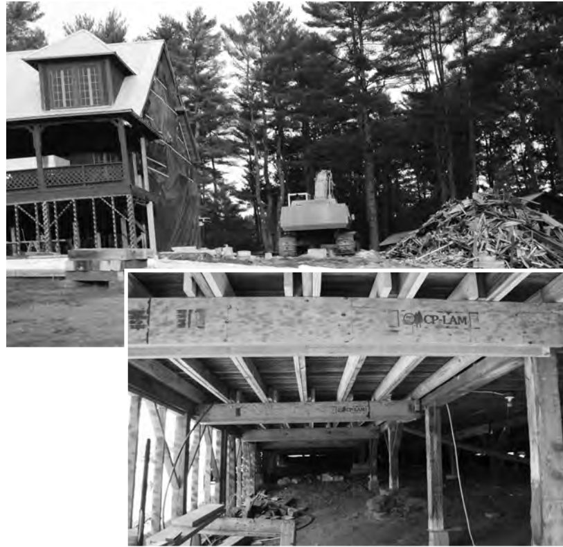
ABOVE: The Lodge with the kitchen and 4 on the Floor removed. BELOW: Looking underneath the lodge with new supports visible.
